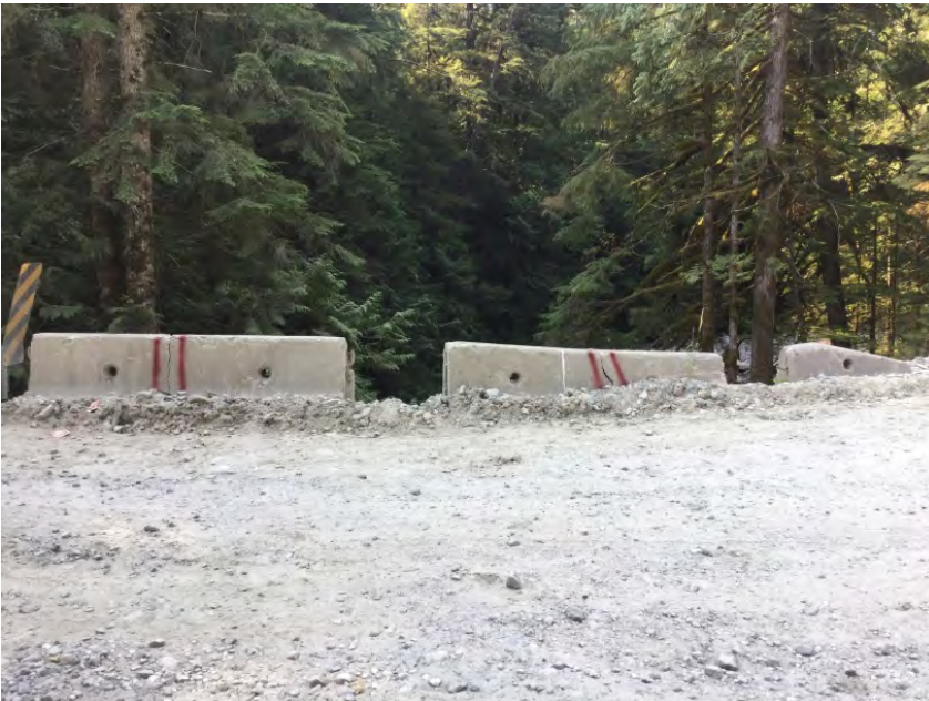
Downstream right bank concrete barriers in poor condition
